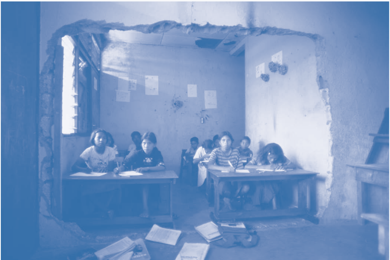
Timor-Leste suffered high levels of infrastructure destruction in the 1999 post-referendum violence.
